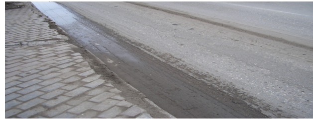
Figure 2 - The result of milling the protrusions during the power circuit control
